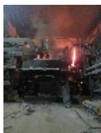
EAF Transformer Monitoring
